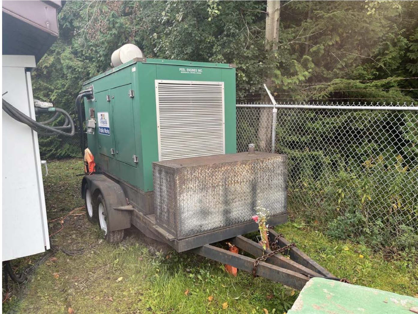
C:\Users\SPihe\PIctures\Well 6\Portable Generator.jpeg
