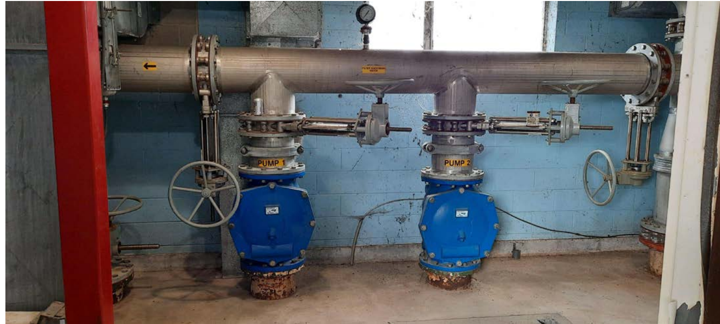
Backwash return pumps
