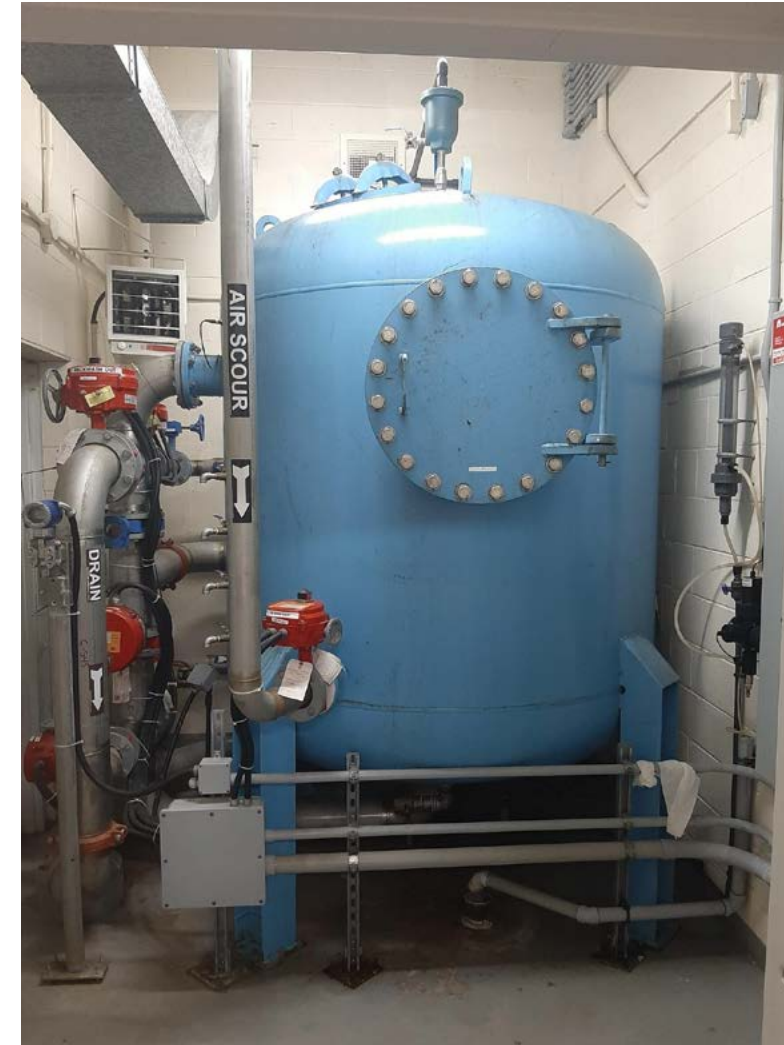
Well 8B/8C Filter Vessel
