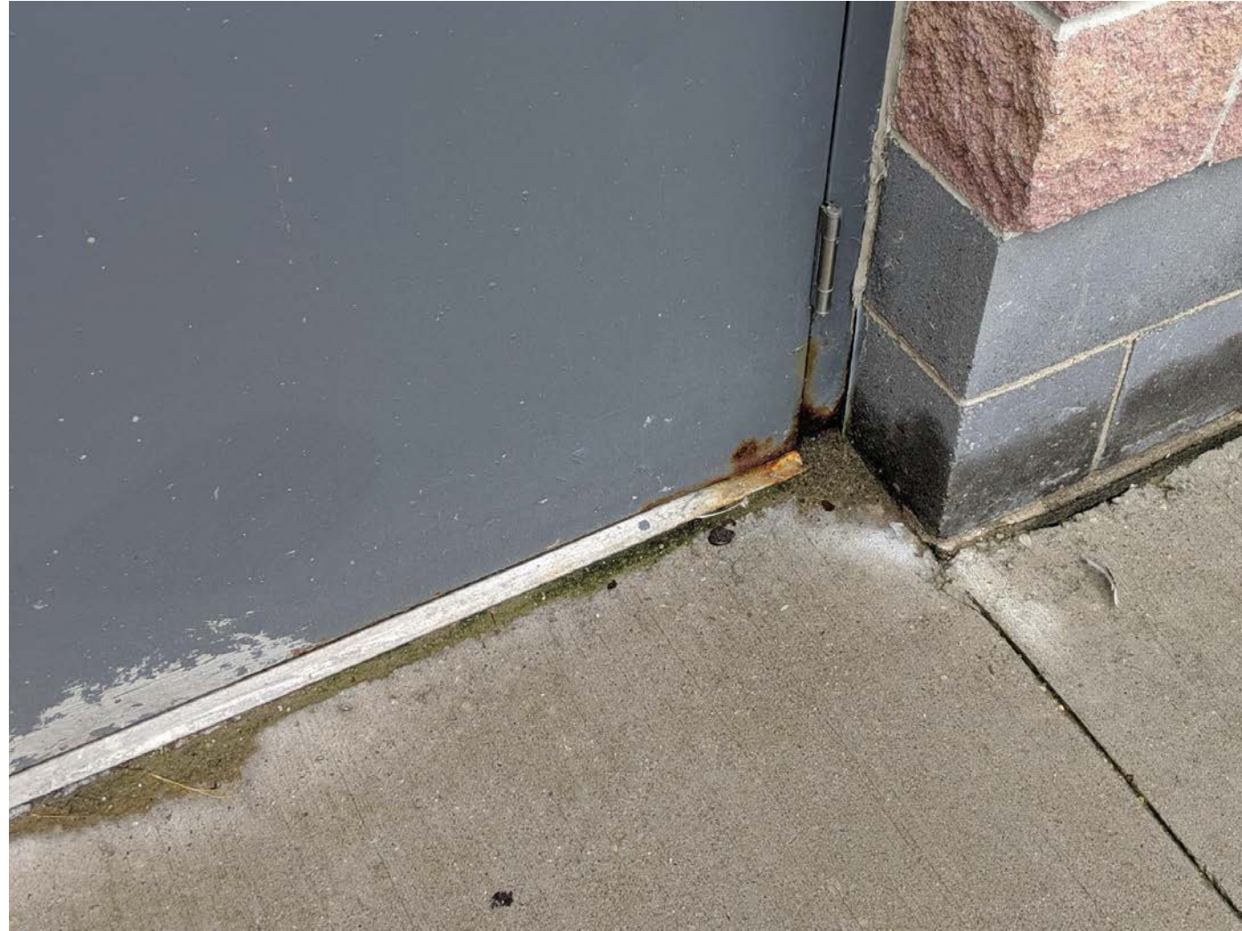
C:\Users\ccosgrove\Town of Orangeville\Facilities - Recreation Facilities\Capital Budget Pictures 2020\Alder Exterior Door 2.jpg
