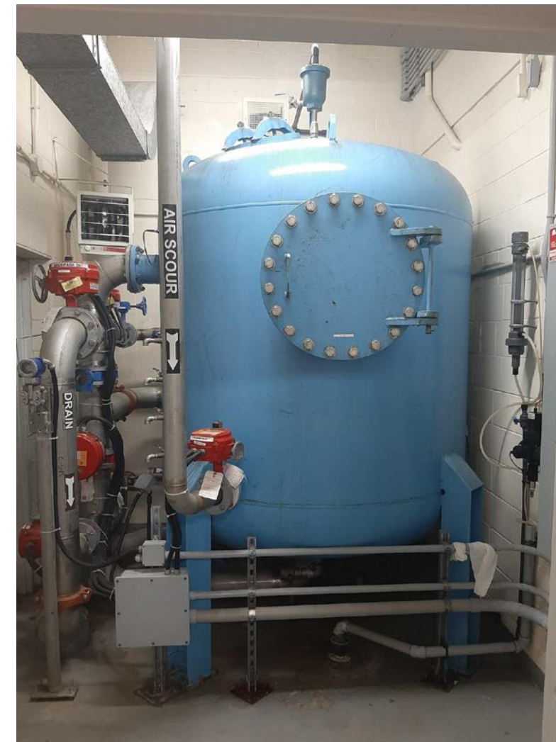
Well 8B/8C Filter Vessel
