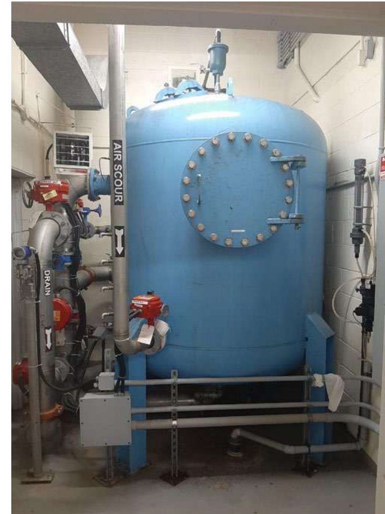
Well 8B/8C Filter Vessel
