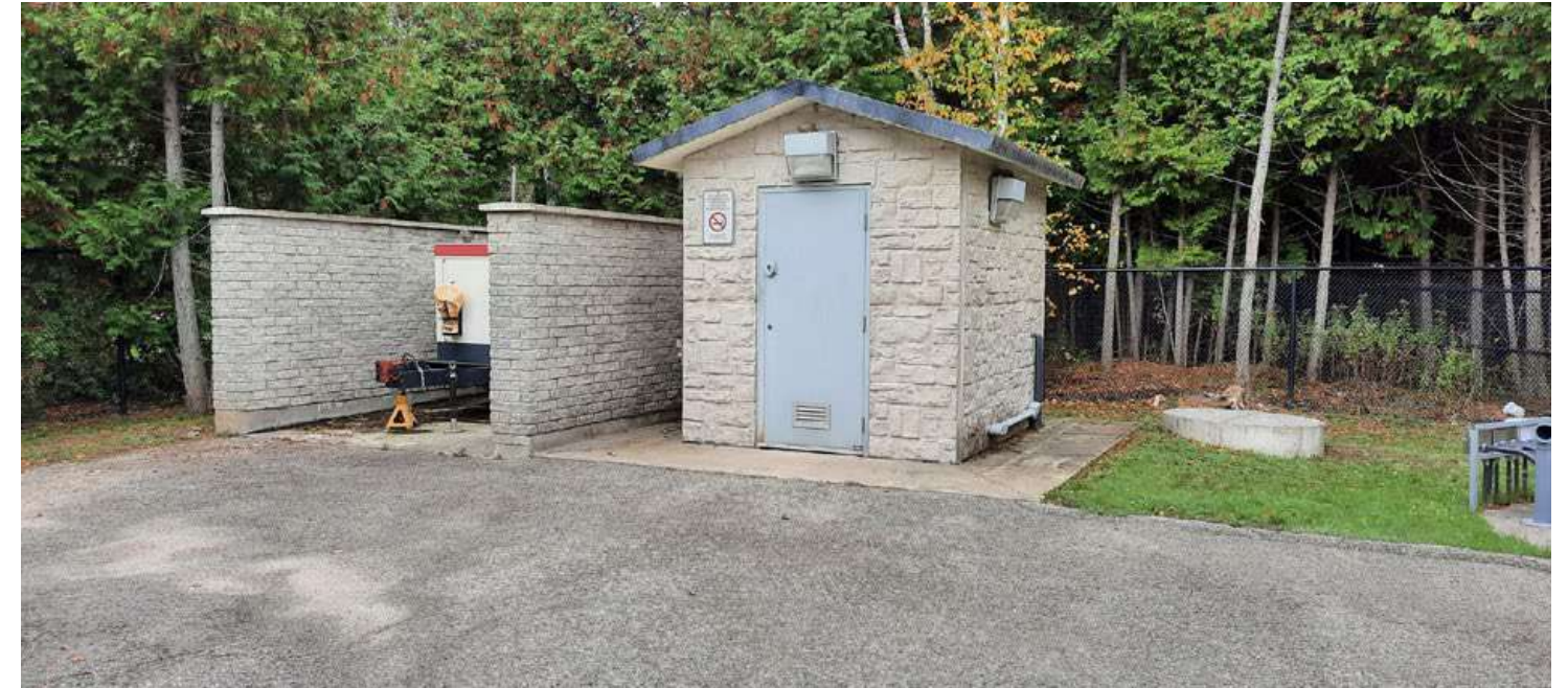
Young Court Sewage Pump Station
