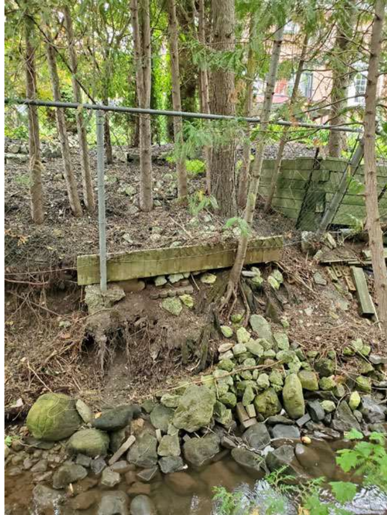
C:\Users\lccosgrove\Documents\2022 Budget pictures\Monora Creek washout 215 Kensington Place\Monora Creek 2.jpg
