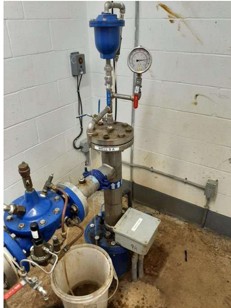
Well 9A - Wellhead
