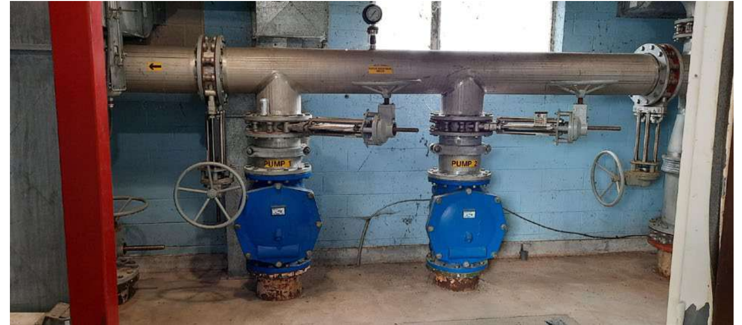
Backwash return pumps
