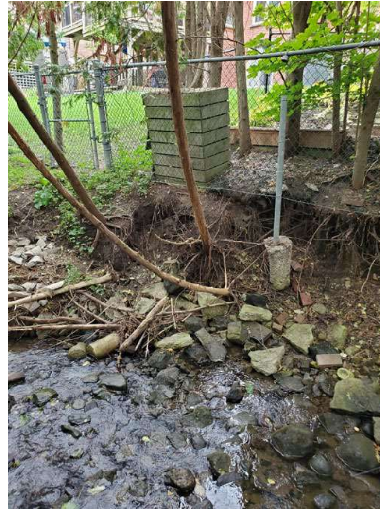
C:\Users\lccosgrove\Documents\2022 Budget pictures\Monora Creek washout 215 Kensington Place\Monora Creek 3.jpg
