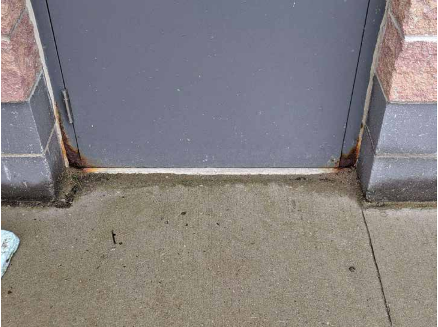
C:\Users\ccosgrove\Town of Orangeville\Facilities - Recreation Facilities\Capital Budget Pictures 2020\Alder Exterior door 3.jpg
