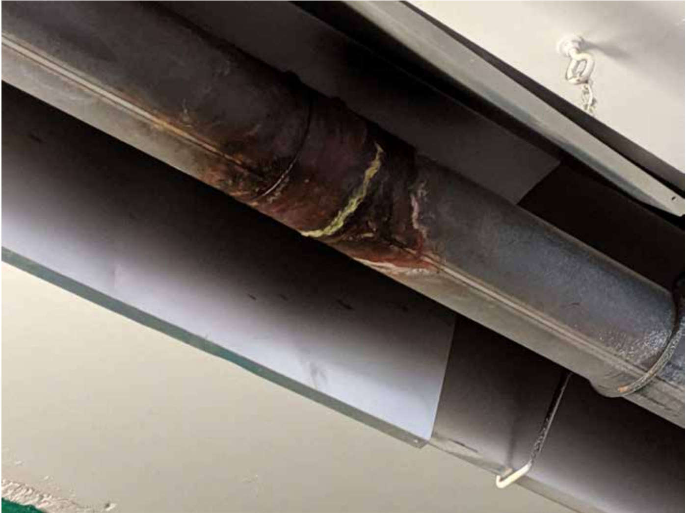
C:\Users\ccosgrove\Town of Orangeville\Facilities - Recreation Facilities\Capital Budget Pictures 2020\Alder Green Rink Heater three.jpg
