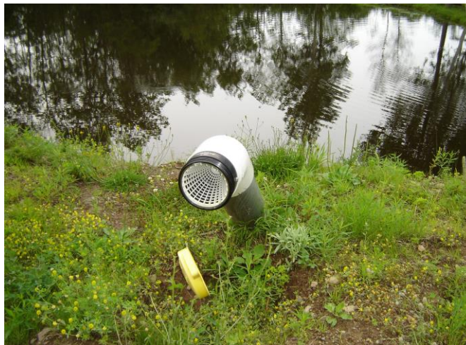
Dry Hydrant on a pond
